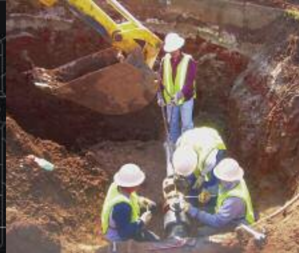
Relocation of natural gas, as well as water and electric services, continues along Governors Drive.
