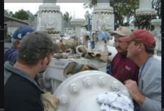
Gas meter technicians train on removing a turbine from a turbine meter for calibration as part of the regular maintenance program at this city gate station.
